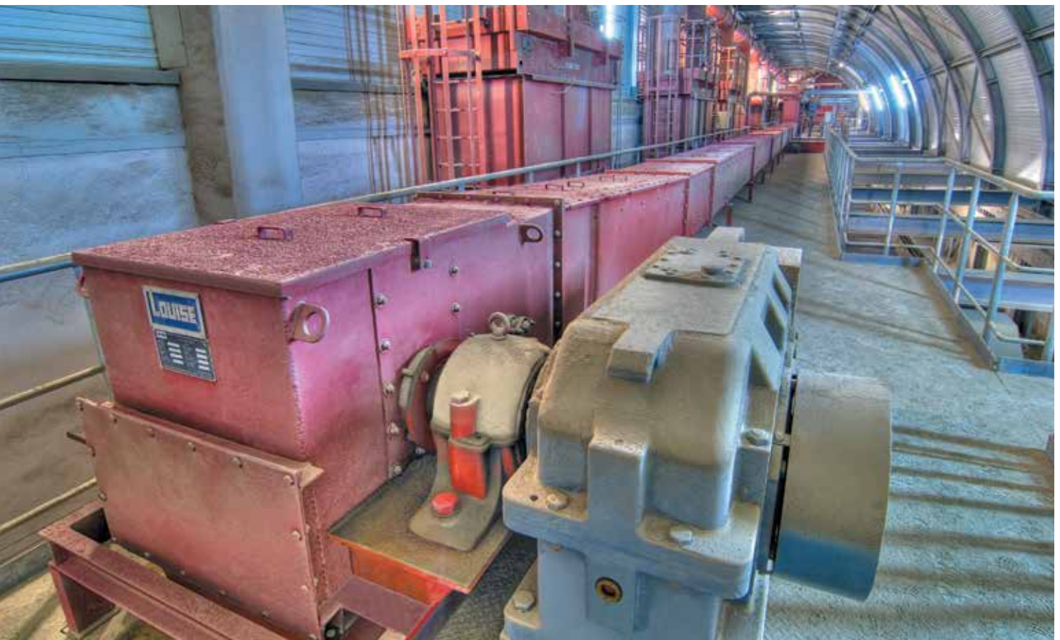
Distributing bulk materials into a battery of silos
