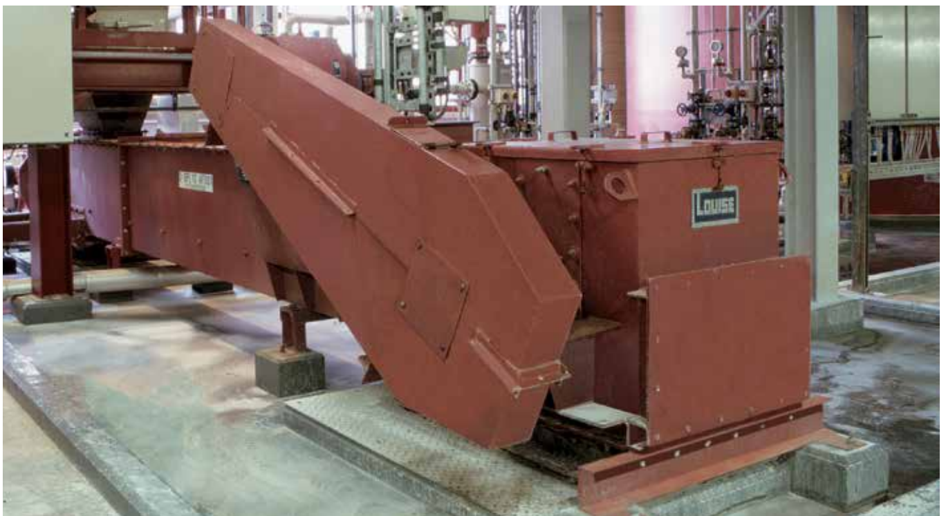
A double-strand Chain Conveyor loads FGD Gypsum from the flue-gas desulphurisation into the storage silo
