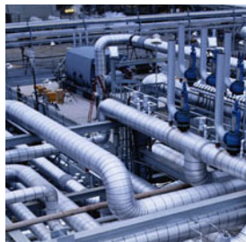
PGW delivers the Natural Gas from the city gate to the burner tip
