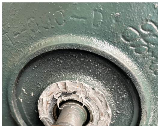
A copious amount of high-quality gray sealant was used when installing the new seal
