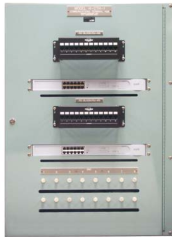
Model H-CTH-1 Communications Terminal Hub
