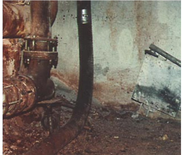
Old ceramic, refractory-type elbow is shown above. Material blown out from frequent plug-ups can still be seen on the floor and pipes.
