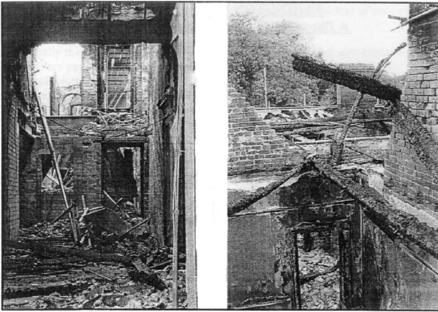
The devastated remains of the House after the fire (above)
