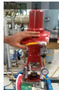
Valve position controller
